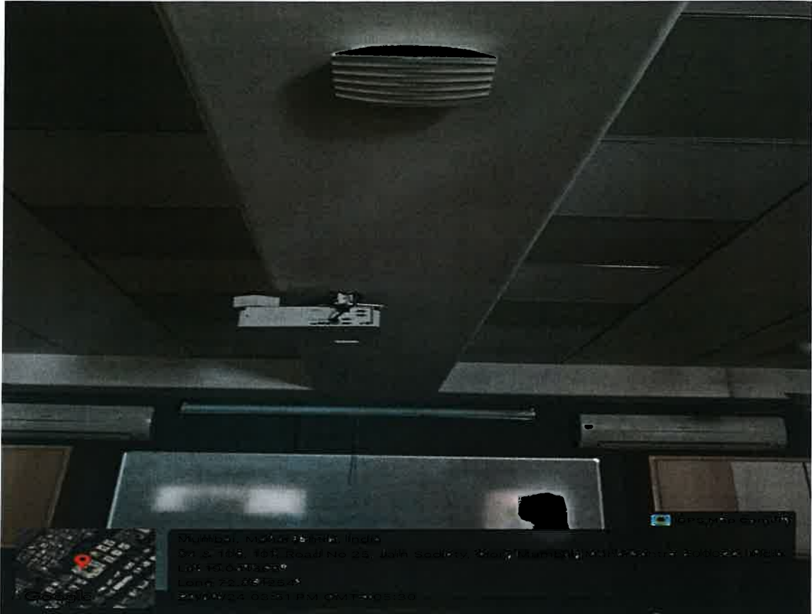
IT Lab – LAB NO 4 - installed since 2018-19.
