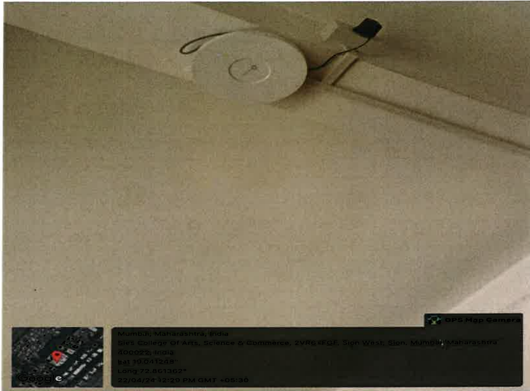
Ground Floor - installed since 2023-24.
