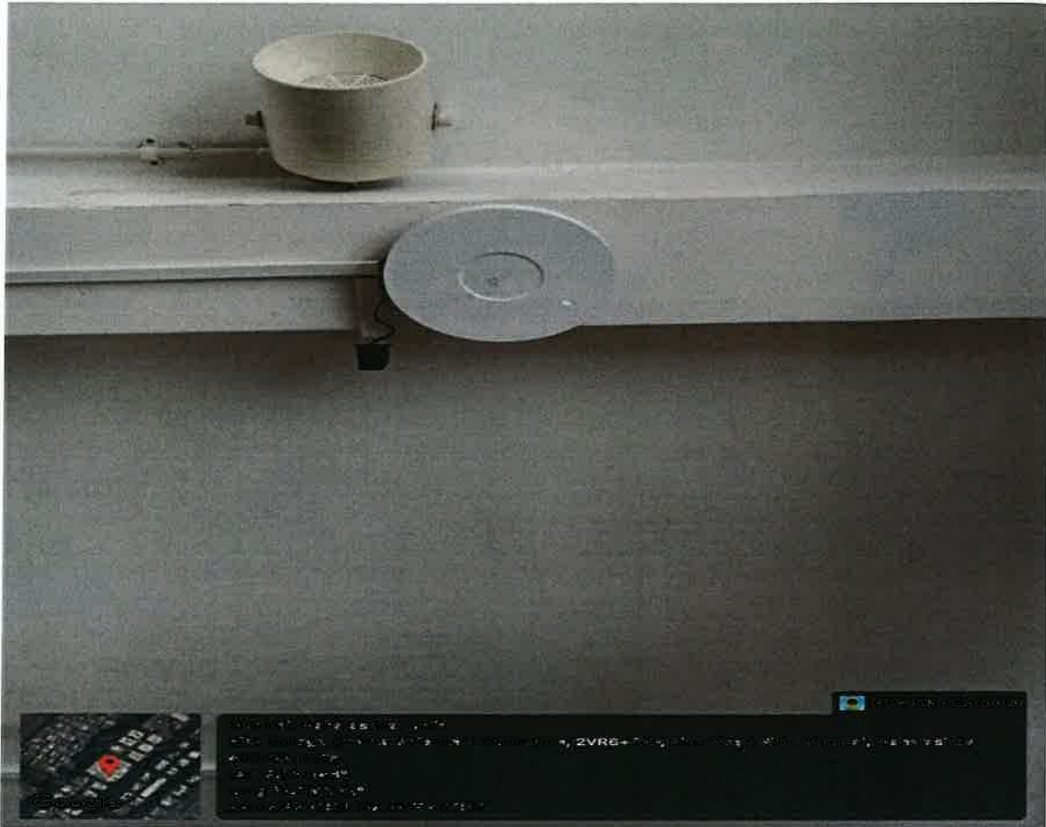
Ground Floor - installed since 2023-24.
